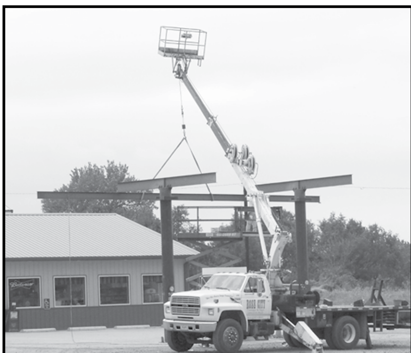
During the last week, crews worked to put up the new canopy over the gas pumps at Allen's Countryside Gas & Grocery station on Highway 9.
